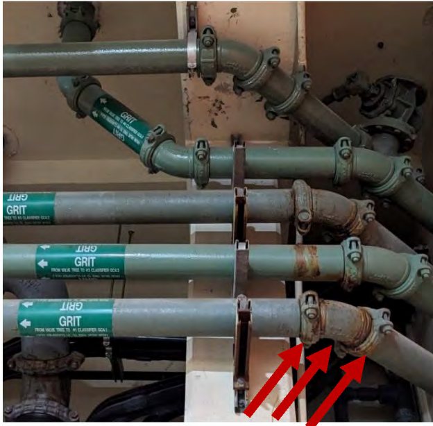
Figure 1: Victaulic grooved fittings and couplings on grit pipes
