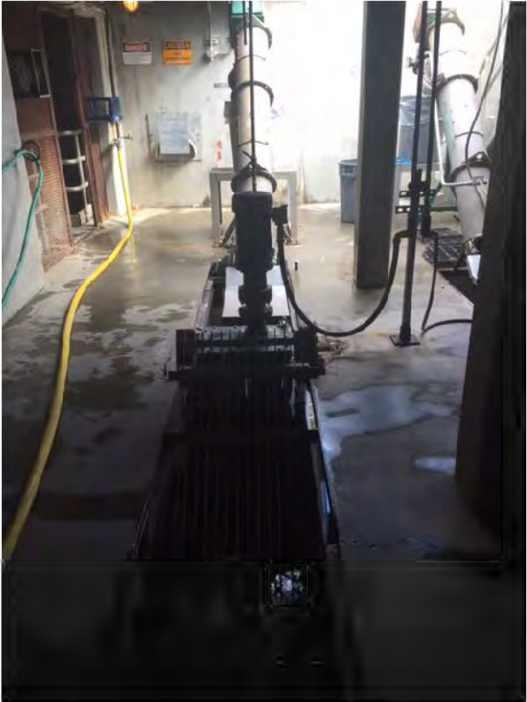
Photo 1: Field Photograph of existing channel grinder and auger system to be replaced
