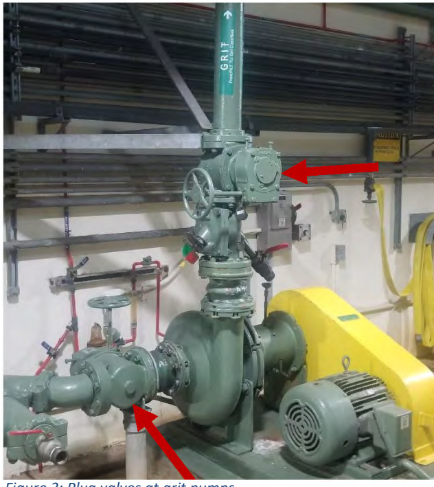
Figure 3: Plug valves at grit pumps
